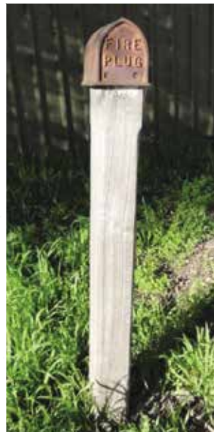
Marker identifying buried Fire Plug.
